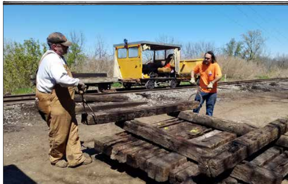
On May 1, Track and ROW Supt. David Kehrer and volunteer Justin Carmona stack old ties to recycle as dunnage, helping to clean up from our tie replacement project in April.
