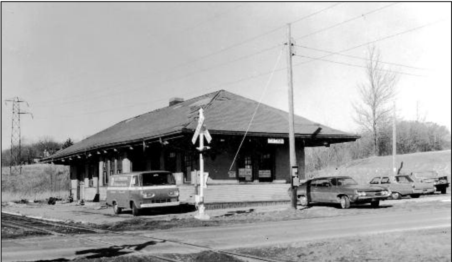
HUMBLE BEGINNINGS: Rochester Chapter volunteers were hard at work in 1971, making desperately needed repairs to the roof and subfloor of the old Erie Railroad depot purchased with the intention of creating a railroad museum. While so much has changed in the last 30 years, what hasn't changed is our organization's pride and determination. Here's to a happy and successful 2011! PHOTO BY RICHARD BARRETT, RGVRRM COLLECTION
