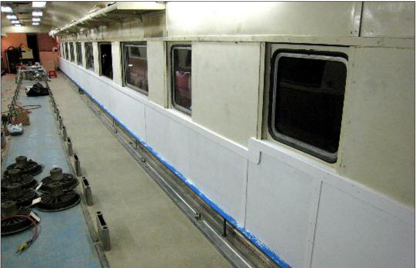
PROGRESS IN COACH 2567: More progress has been made on the interior restoration of ex-New York Central Empire State Express coach #2567. Chris Hauf and his painting crew has been busy over the last few weeks. On September 7, the east side new lower wall was primed in preparation for finish painting. PHOTO BY CHRIS HAUF
