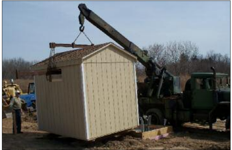
The Chapter purchased a pre-constructed building from Wood Tex in Himrod, NY. The building was delivered on 3/30 and volunteers moved the building onto the foundation on Saturday 4/3. Chad Timothy used the Chapter's Army wrecker crane to position the building onto the foundation designed by member Bob Mader. We expect our contractor to make all connections and soon have water flowing. PHOTO BY JEREMY TUKE
