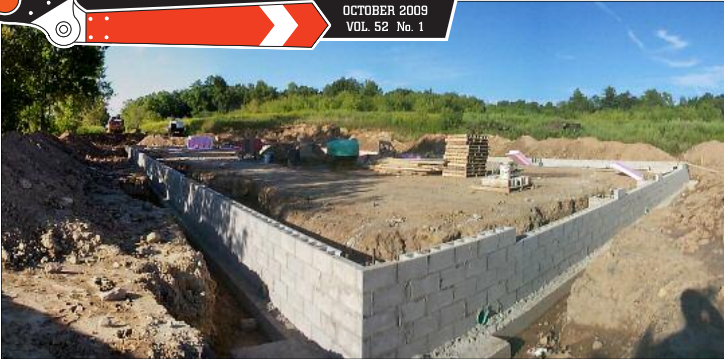
WAY BACK IN THE TWENTIETH CENTURY, Rochester Chapter was engaged in the construction of the Restoration Building, as seen in this 1998 photo. While the structure has been completed and we have temporarily moved in, the job is far from done. In order to have a functional restoration shop, we must complete and install the inspection pit, a full concrete floor, lights and more. You can help by contributing to our Annual Fund Drive. Your support today will help ensure our museum's future for years to come. Visit www.rgvrrm.org for more details. PHOTO BY CHRIS HAUF
