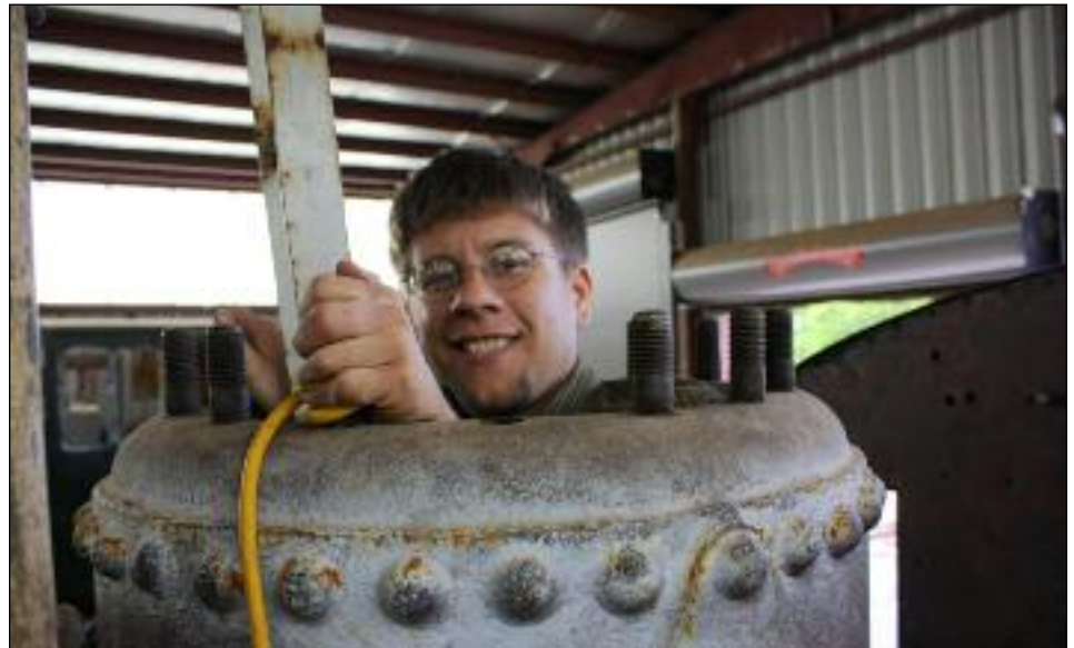
Motive Power Dept. Superintendent Joe Nugent emerges from the steam dome of former Brooklyn Navy Yard 12. Joe assisted Ron Amberger in taking thickness measurements of the steam locomotive's boiler. Those measurements will be used to calculate potential maximum operating pressure, with confirmation from The Strasburg Railroad's chief mechanical officer. PHOTO BY RON AMBERGER
