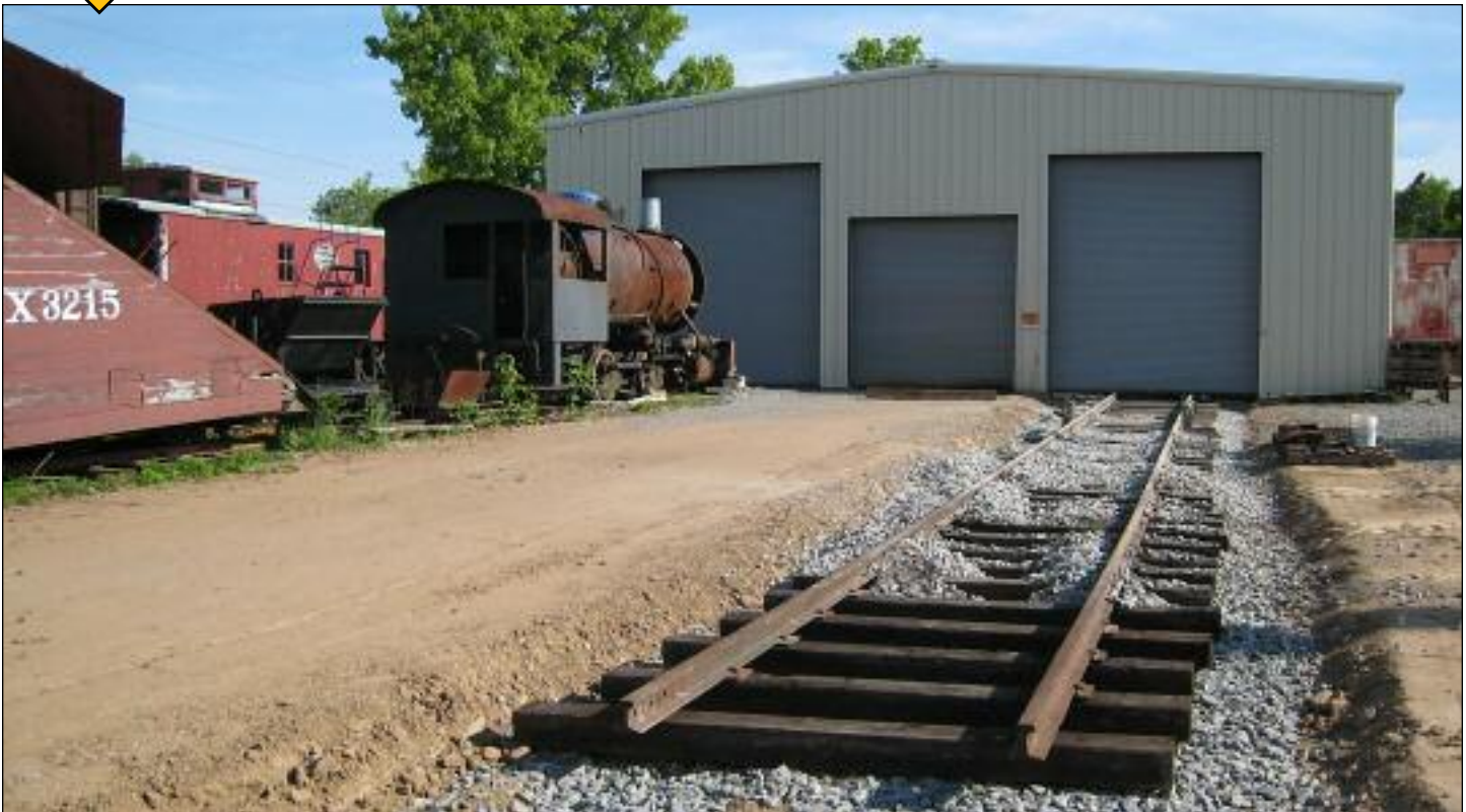
Track 8 now extends through the shop and out the south end. Further expansion will give us greater flexibility in storing our railroad equipment that is not in use or awaiting restoration. By the time you read this, you may see even more extended track! PHOTO BY CHRIS HAUF
