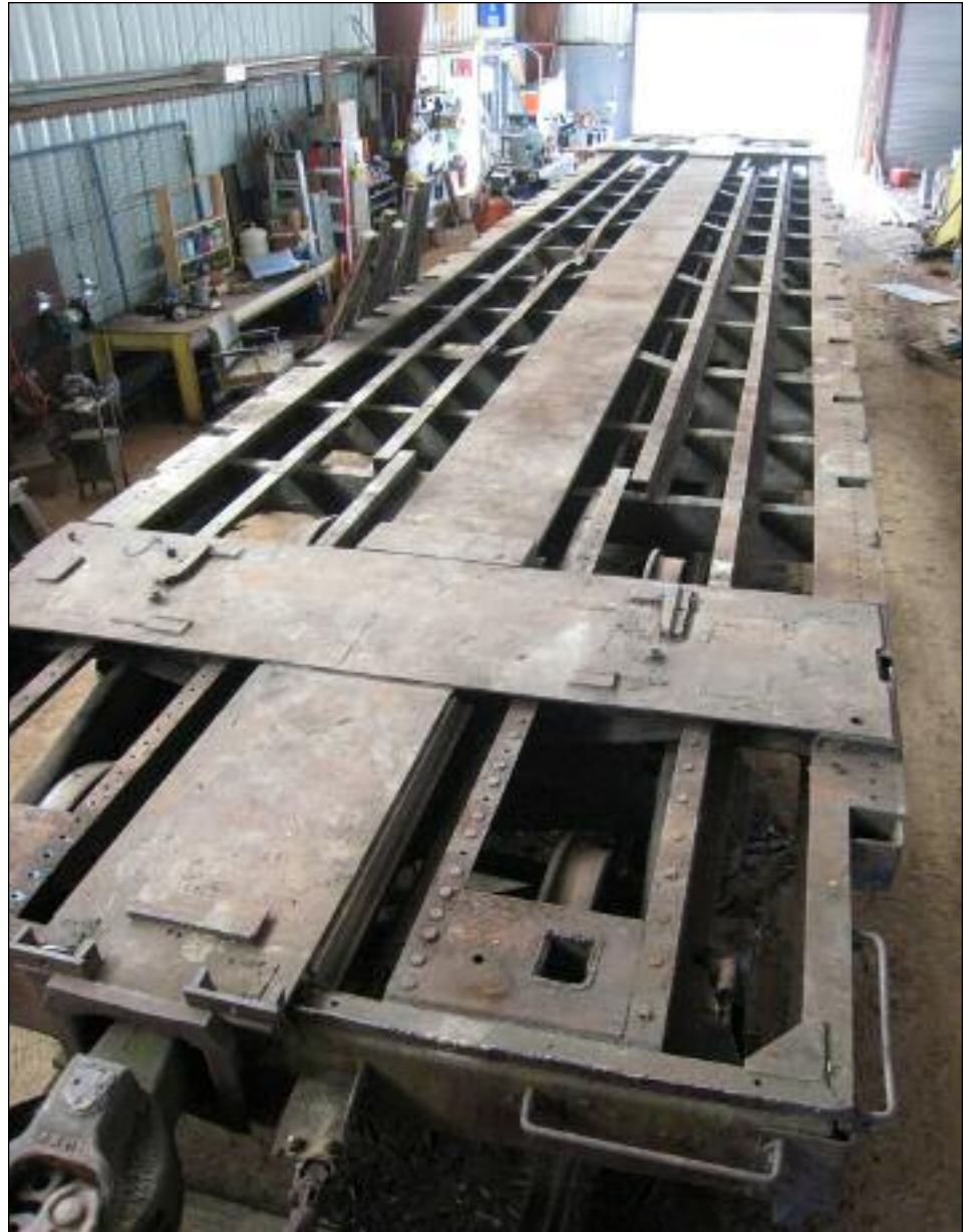
This is what a flatcar looks like naked. The old decking has been removed, now work can begin on repairs and installing a new deck. PHOTO BY CHRIS HAUF
