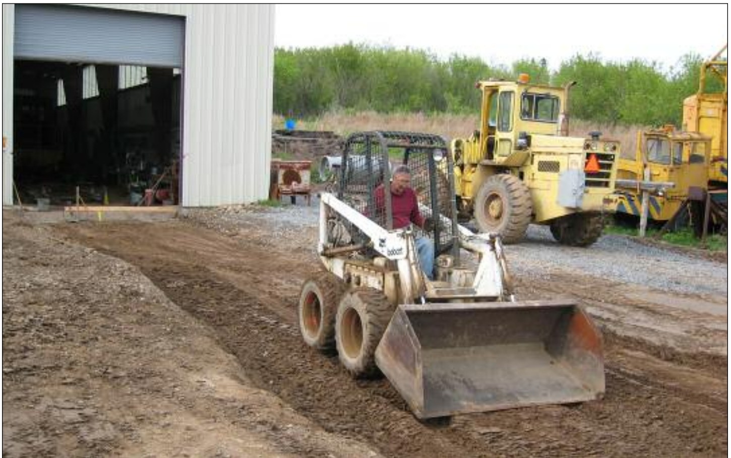
BEFORE THERE WAS TRACK 8, there was dirt to be graded and leveled. Our fleet of heavy and light construction equipment has been very valuable to us over the years, allowing us great flexibility when it comes to our construction projects. PHOTO BY CHRIS HAUF
