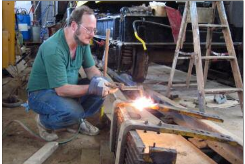
Careful attention to cosmetic detail signals that the rebuild of our 45-ton siderod switcher is nearing an end. Volunteer Kevin Klees is seen heating one of the foot boards from RG&E 1941 prior to straightening the support bars. PHOTO BY RON AMBERGER
