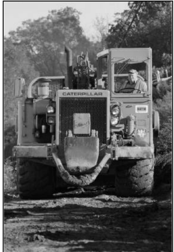
John McDonald has the Cat 627B scraper under control as he completes a pass and brings the big machine alongside the Restoration Building on his way to dump another load of dirt in the fill area. [Caption and photo by Chris Hauf]
