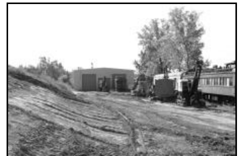
After the Big Dig: On October 2, 2005, the story has drastically changed. The dirt is gone and now the entire north end of the building can clearly be seen. The bank still needs to be trimmed back a little further to the east to allow for Track #8 to be installed, but will go fast, and with some grading and drainage work, we will be clear for the installation of the switches and tracks necessary to get our Restoration Building connected to our railroad!
