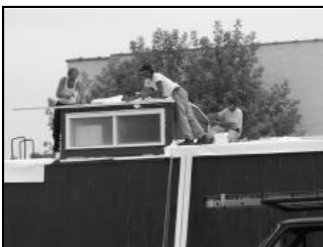
Workers from the roofing company had previously applied the rubber membrane material. Here, they returned to do the final trimming.
