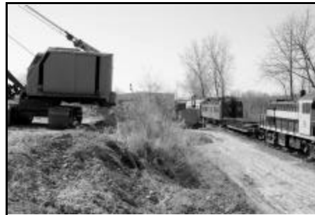
Before the Big Dig: On April 16, 2005, there was still a mountain of dirt to be moved at the north end of the building as only Restoration Building's roof can be seen over the dirt in this shot looking south.
