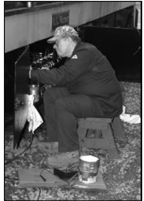
Jim Johnson takes care of the final step by hooking up Eastman Kodak Co. GE 80-tonner #6 new batteries. With new batteries, the engine was checked over and returned to service. Thanks to all that donated to allow us to buy these batteries. ( Chris Hauf photo )
