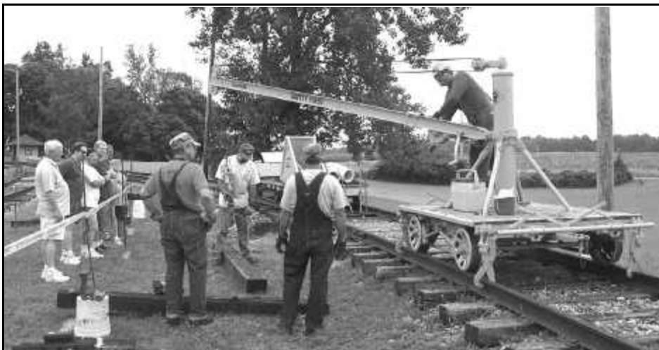
On August 3rd, the joint museum's hosted another special event - "Gandy Dancer Day", which demonstrated how the railroad track work was and still is performed around the museums. Here we see our gandy dancers using the newly restored Fairmont track crane to demonstrate the lifting and movement of railroad tie into position to a group of museum visitors. In the background is Randy Bogucki's recently constructed ballast cleaner. (Photo by Chris Hauf)
