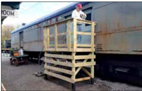
ABOVE LEFT: Jeremy Tuke and Otto Vondrak completed construction of the new platform entrance for the Lackawanna baggage car exhibit on October 23. New stairs will be built in 2021.
