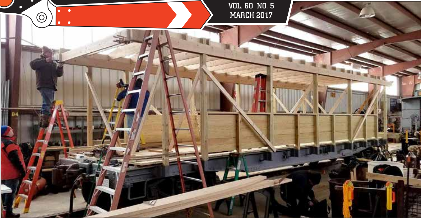
Not quite Despatch Shops, but volunteers are making great progress on our new open-air rider flatcar. Built on the frame of Lowville & Beaver River No. 23 (ex-U.S. Army), this new car will more than double our passenger capacity for special events. OTTO VONDRAK PHOTO
