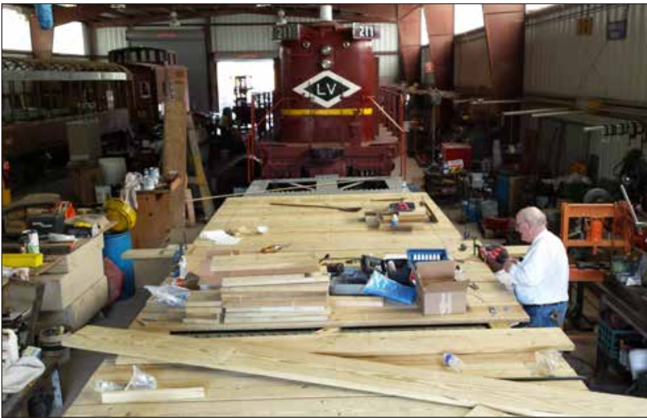
LEFT: The wood deck is nearly complete on our ex-Army flatcar. The next step involves installing benches, sides and a roof. The benches have already been constructed. Your museum needs your help to raise $3000 to complete the next phase of construction. Can you help? Our goal is to have our new open-air rider flatcar ready for testing this year. The addition of this car will give us increased capacity for our fall busy season.
