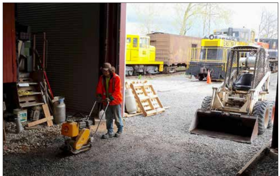
Adam Lloyd compacts another layer of crusher run brought in by the Bobcat loader at right to prepare the base for the next pour of concrete inside the Restoration Shop. Not only does the concrete floor make a cleaner environment, it makes it easier to work and move materials inside the shop.
