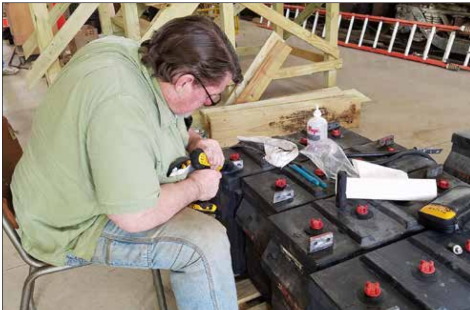
LEFT: Jim Johnson cleans the terminals and checks the wire leads on the locomotive batteries donated by Livonia, Avon & Lakeville Railroad. While these batteries are a few years old, they still have plenty of life left in them for our purposes. The batteries will be used in LA&L No. 20, which will be reactivated this fall. MIDDLE: On July 11, Dave Luca and Charlie Marks place grab irons to mark where to drill holes for mounting hardware on the Buffalo, Rochester & Pittsburgh caboose. BELOW LEFT: Giving “yard work” a whole new meaning Mike Dow, Syeria Dow, Adam Lloyd, and Dave Scheiderich inserted several new ties around Switch No. 5 on July 4.
