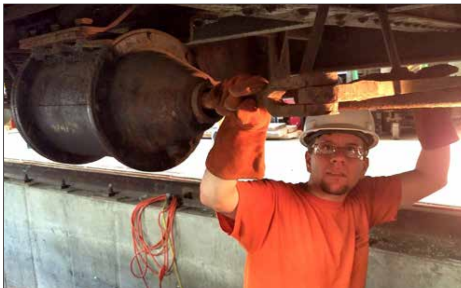
Joe Nugent cleaned and replace the piston in the air brake system under the LBR 23 open-air rider car on July 11, while Rob Burz worked to reconnect the hand brakes.
