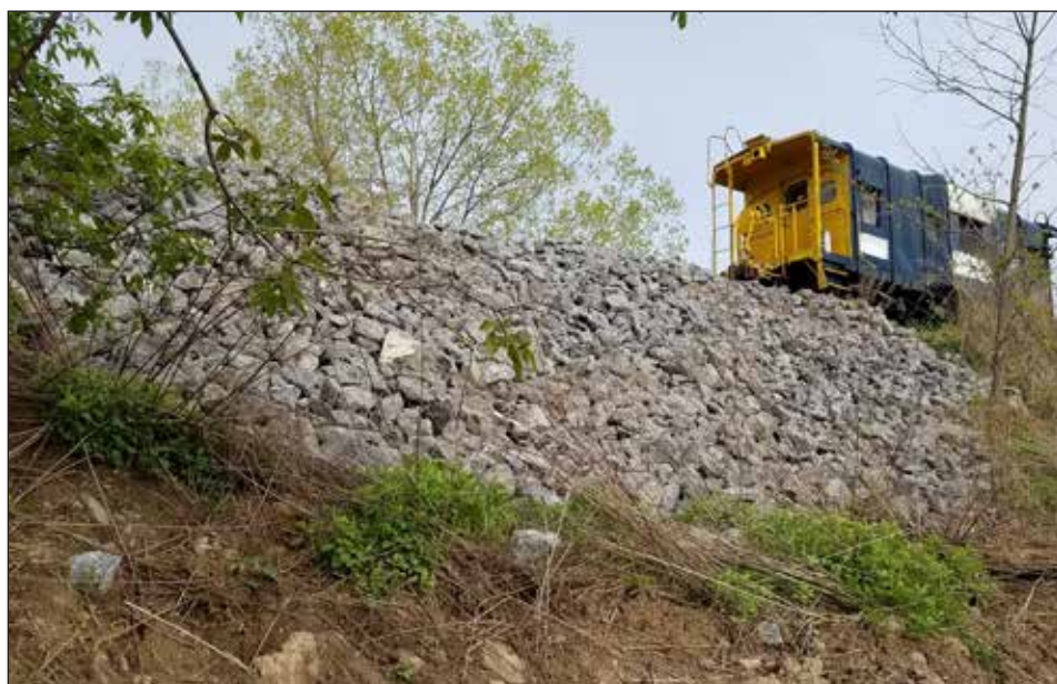
A mudslide was discovered on April 8 alongside the new Track 6 extension. Repairs were made on April 10, thanks to six truckloads of rip-rap coordinated by volunteer Scott Gleason.
