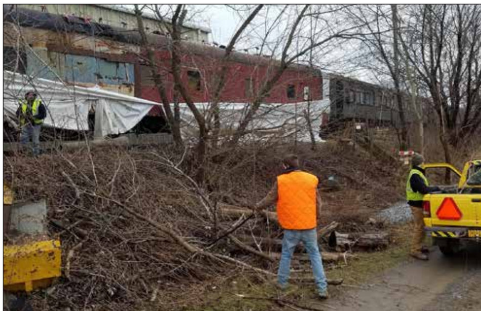
Adam Johnson (LEFT) and his son Tyler (CENTER) help Mike Guglielmo (RIGHT) load branches and debris for disposal during our Clean Up Day on April 1. Wind storms destroyed the shrink wrapping on the Pine Falls and caused minor damage elsewhere.
