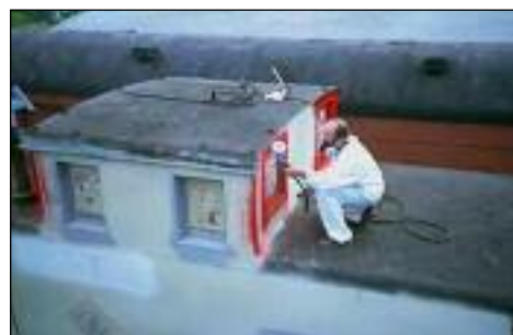
Many folks had a hand in C254's restoration from Conrail blue to Erie red. Volunteer Lynn Cross applies the first coat of "American LaFrance Red" to the cupola of the caboosie during a August, 1994 work session. PHOTOS BY CHRIS HAUF
