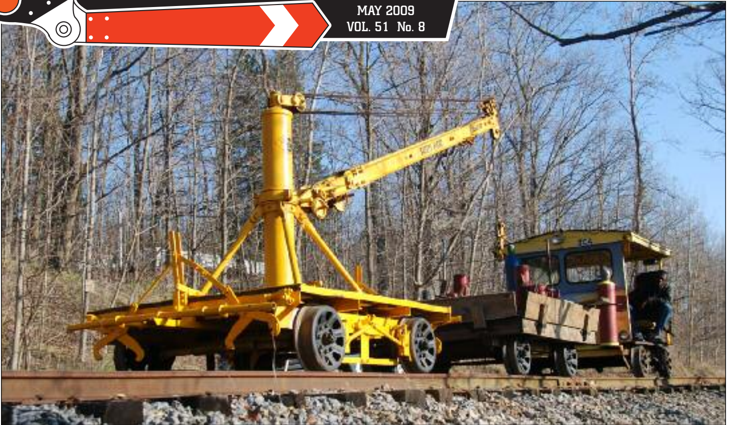
TC-4 powers a short work train consisting of our Fairmont crane and a flatcar up the mainline, north of Switch 6. Track patrols throughout the off season have worked to keep our lines in top operating condition, getting ready for the 2009 museum season. PHOTO BY DAVID SCHEIDERICH
