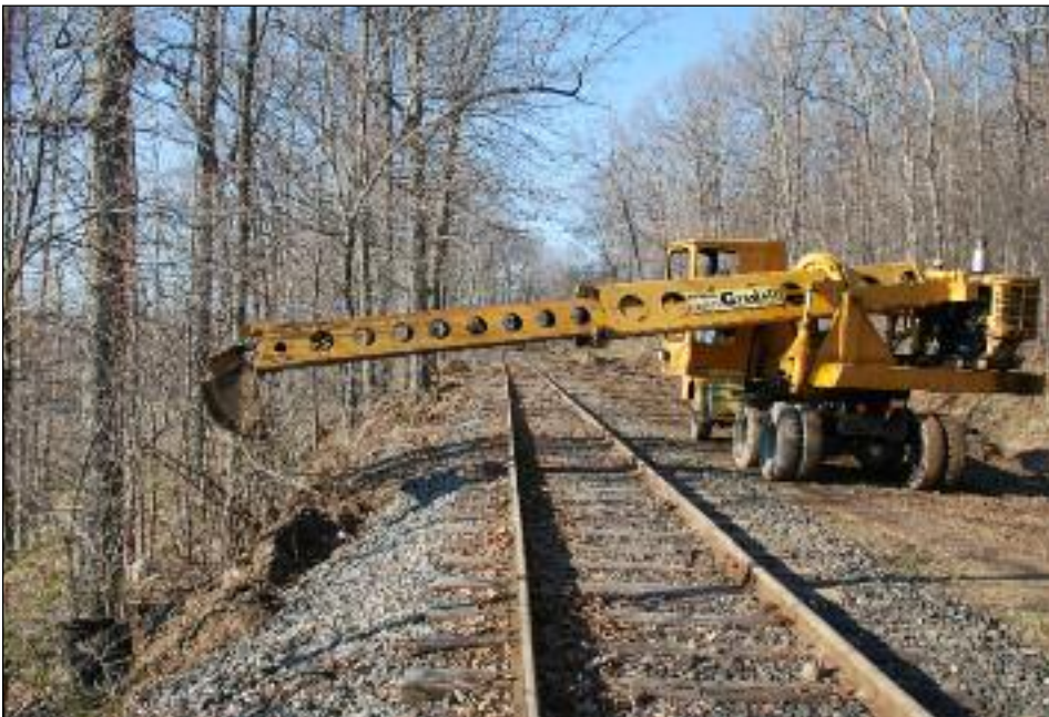
THE GRADALL AT WORK: Our Gradall machine has proved to be a useful tool around our museum grounds, seen here clearing obstacles north of Switch 6. We have also been using the Gradall to help with our various drainage projects around the property. PHOTO BY DAVID SCHEIDERICH
