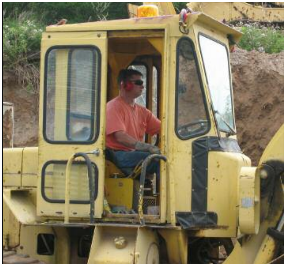
Scott Gleason has the controls of the museum's Trojan loader as more dirt is moved from the north end of the building to the south end. There are plenty of opportunities for volunteers who wish to learn more about working with heavy equipment. PHOTO BY CHRIS HAUF
