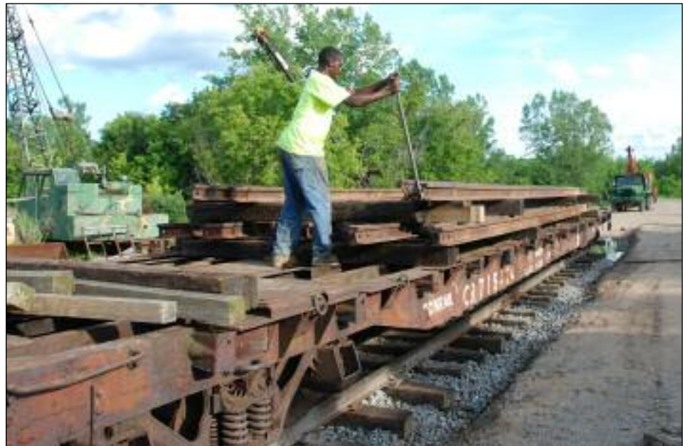
Luther Brefo coaxes a rail into position on the stack of material that is being prepared to move to the work site where our new excursion set storage siding will be built. PHOTO BY DAVID SCHEIDERICH
