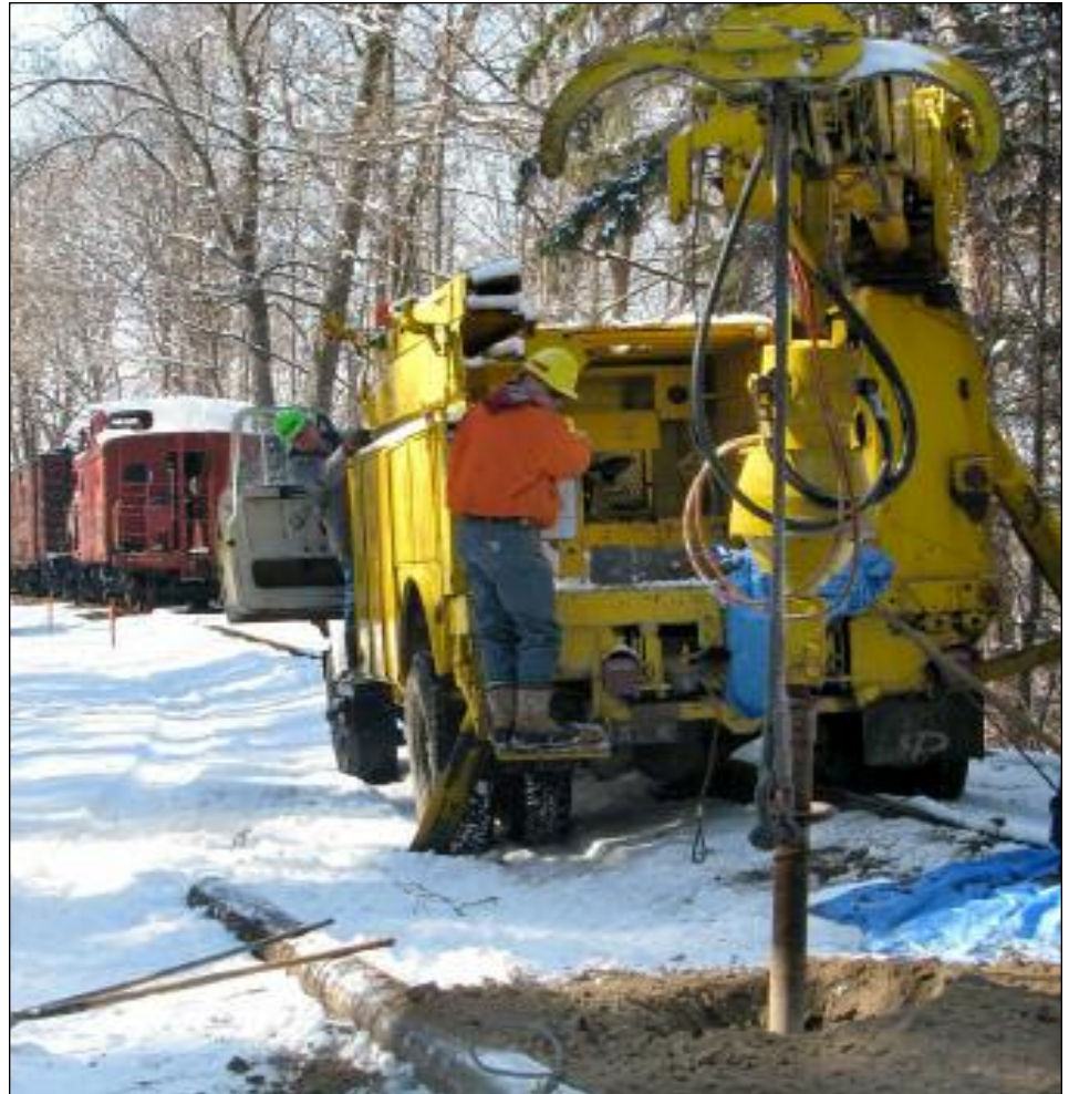
SETTING NEW POLES: Following on a successful extension of their trolley wire last year, the NYMT with assistance from R&GVRRM volunteers and equipment took the next and biggest step, planting the poles to extend their trolley wire to the end of the NYMT property at approximately milepost 0.5. Here we see R&GVRRM volunteers, Scott Gleason and Dan Waterstraat, working the R&GVRRM's auger truck to set the second to last pole. The R&GVRRM's railroad equipment stored on the mainline can be seen in the background. PHOTO BY CHRIS HAUF
