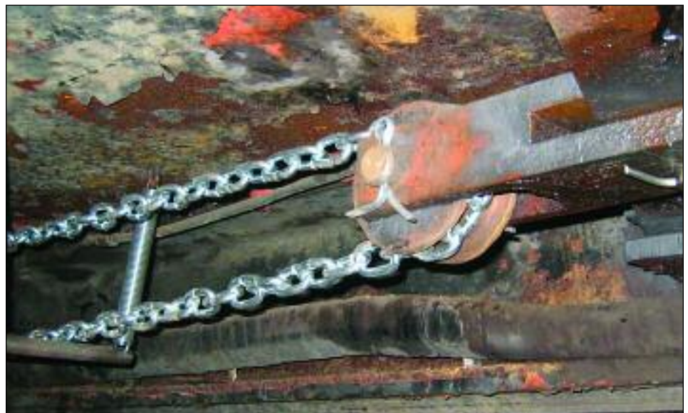
Thanks to our Motive Power Team, the hand brake mechanism on ex-Eastman Kodak Company 80-tonner #6 has been completely renewed with cleaned pulleys, brand new pins machined by Kevin Klees, new spring hangers for the chain, and a brand new chain. With the challenging topography of our demonstration railroad, effective hand brakes are a must. PHOTO BY CHRIS HAUF
