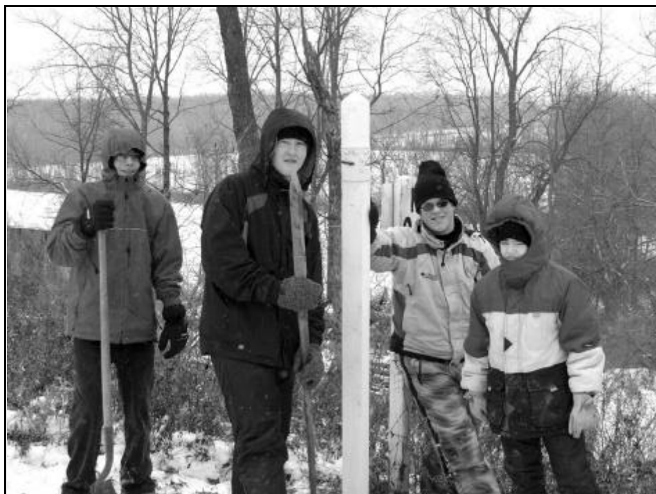
Jason Marks has undertaken an Eagle Scout project at the R&GV RM. Jason is installing all new mileposts and station markers along our demonstration railroad since most of our original mile markers, built by Neil Bellenger nearly a decade ago, have been stolen or vandalized. Here Jason (center left) works with his crew while installing a 4x4 post near Switch #6 this past December. (Chris Hauf photo and caption)
