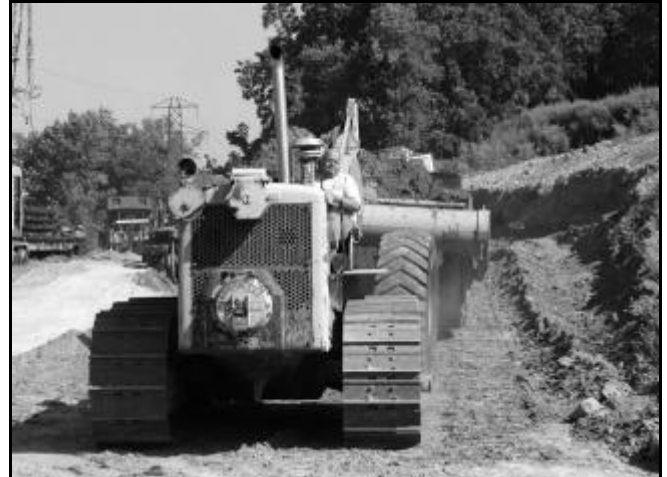
John McDponald pilots the Cat D8 tractor and tractor pan through the dirt with Joe Scanlon pushing on the rear with the Cat D7E dozer. This dig area lines up with the large railroad door on the east side of the Restoration Building [Chris Hauf photo & caption]
