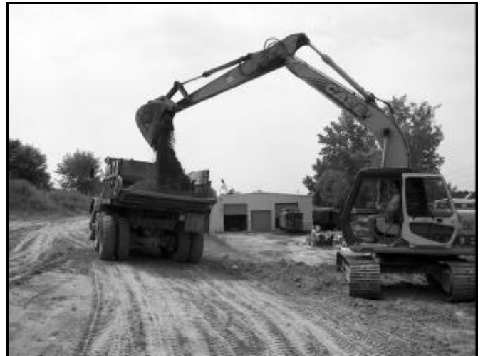
The BIG DIG continues at the North end of the Restoration Building. (Mike Roque' photo)
