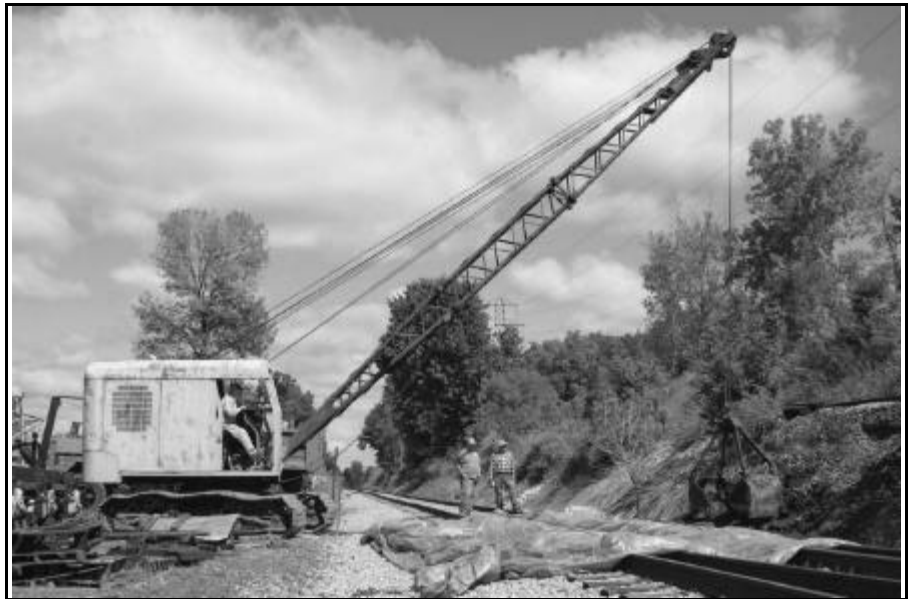
Above: The Northwest crawler crane with its clam bucket eases earth across the LA&L tracks. Note the tracks were protected from 'spillage' by a tarp.
