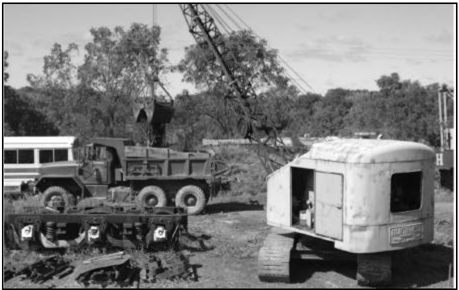
Below: The resulting bucket of earth was transferred to one of the ex-Army dump trucks and hauled to a more suitable location! [Photos by Chris Hauf]
