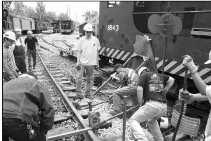
Top: Norm Shaddick has the museum's Jackson tamper working on the rebuild of Switch #5 frog. This unit makes easy work of driving new stone under the ties to give the track a solid road bed.
