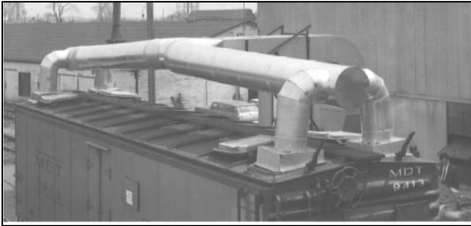
This photograph shows the four ducts, from the dryer, attached to the reefer hatches. (Photo by Harold Crouch)
