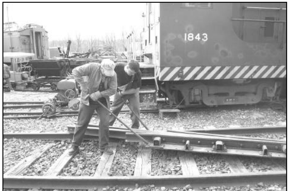
Randy Bogucki and Tony Mittiga put their shoulders into moving the rebuilt frog for Switch 5 into place the old fashioned way with lining bars. Digitig photo by Chris Hauf
