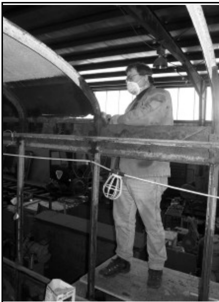
Dave Luca removing the rotten steel roof panels from Car #60. (Chris Photo)
