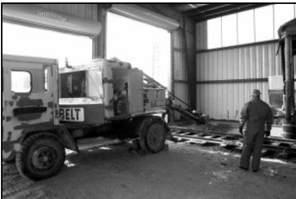
The R&GV RM's Link-Belt excavator starts the dig for the electrical service vault inside the Restoration Building.
