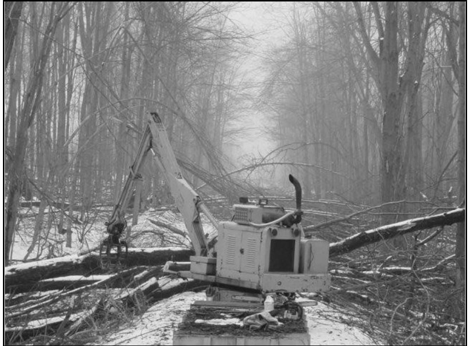
OMID crews work to clear ex-PRR section of mainline of fallen trees following the April 3-4 Ice storm which devastated much of Wayne and Monroe Counties. Photo by Gregg Carpenter
